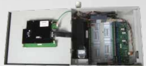
Powered biCoders installed in same enclosure as controller
