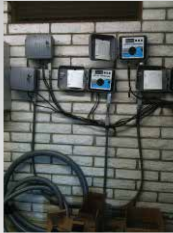
Before: Multiple Controllers
